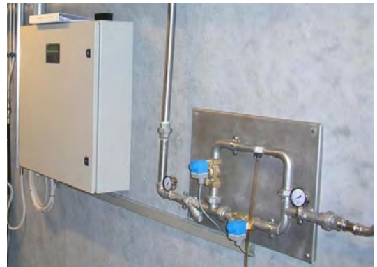
Control Board Automatic CIP cleaning unit.
